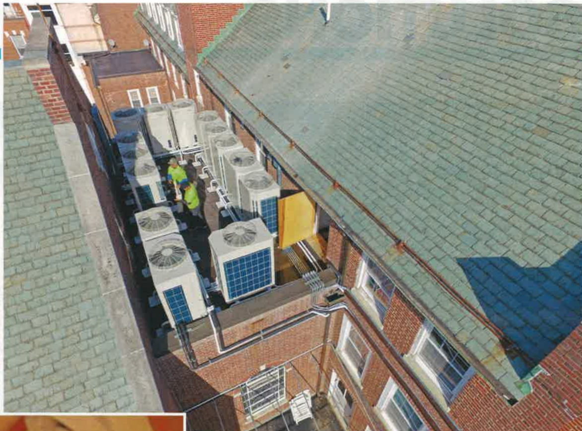
BIRD'S EYE VIEW: Technicians with Brookfield, Connecticut-based Green Star Energy Solutions LLC check the 14 variable refrigerant flow (VRF) condensers mounted on a small roof atop the Convent of St. Dominic in Blauvelt, New York. The facility is the headquarters for the Dominican Sisters of Blauvelt's housing administrative offices.
