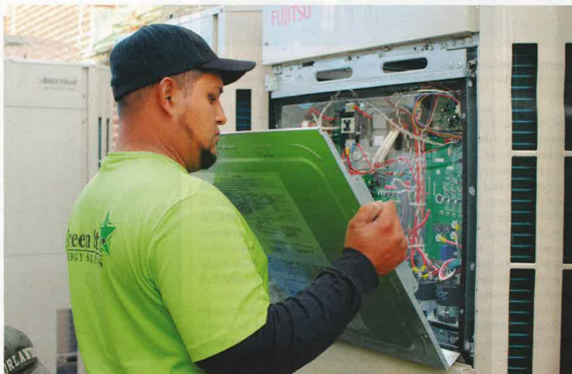
TONS OF COMFORT: In all, 120 ton of VRF heating and cooling capacity is installed to serve the 100,000-square-foot building.
